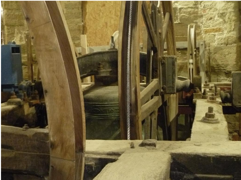
Top: cracking and decay in the frame. Above: eight bolts in one small stretch of 19th-century wood! Old and new materials show the years of changing, patching – and weakening.
